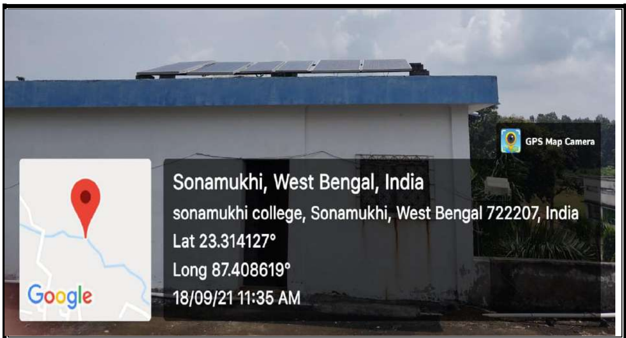
SOLAR PANEL (3 KILOWATT) ON ROOF TOP
